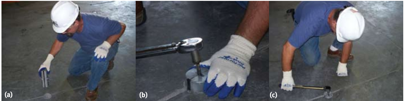
Fig. 2: Steps required to install a device: (a) after removing the core from a core-drilled hole centered over the joint, the split cylinder is inserted into the hole; (b) using a wrench inserted through a hole at its top, an internal screw is tightened to expand the cylinder; and (c) with the cylinder joint aligned with the floor joint and the cylinder top flush with the slab surface, a torque wrench is used to tighten the internal screw to the torsion recommended by the manufacturer
